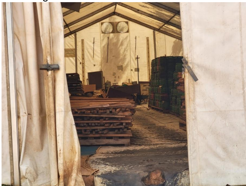
Figure 48: The photo shows a storage unit in Mahama, in which LPG cylinders are stored.
